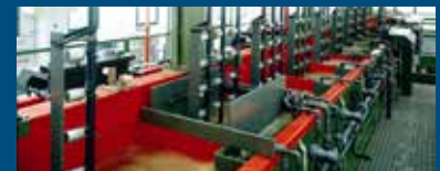
Rectifiers and electro-plating.
