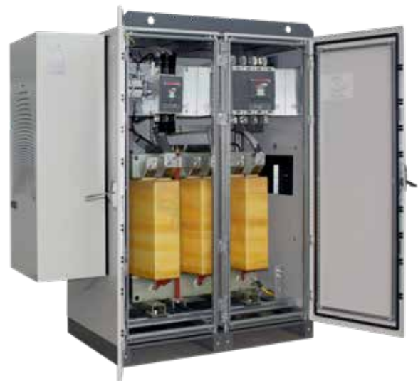
Transformer housed inside an IP54 enclosure with circuit breakers and air conditioners.
