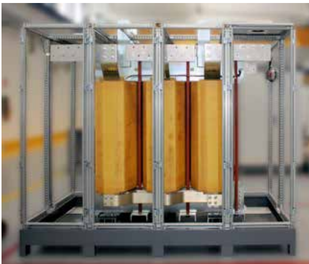
2000kVA transformer within IP21 cabinet.
