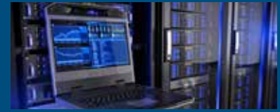
Data center power supply systems.
